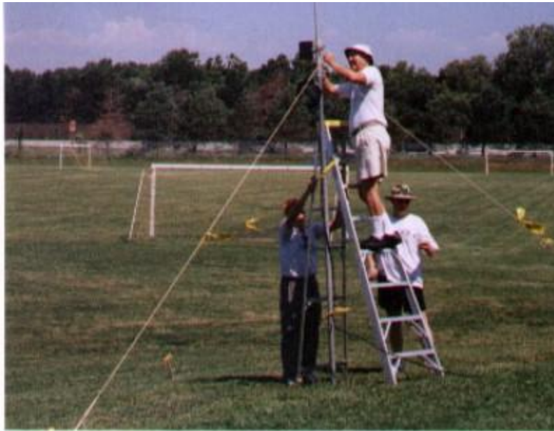
Photo 9: L-R: Stan, Bill (on ladder) and Terry put the final touches on the vertical antenna.
