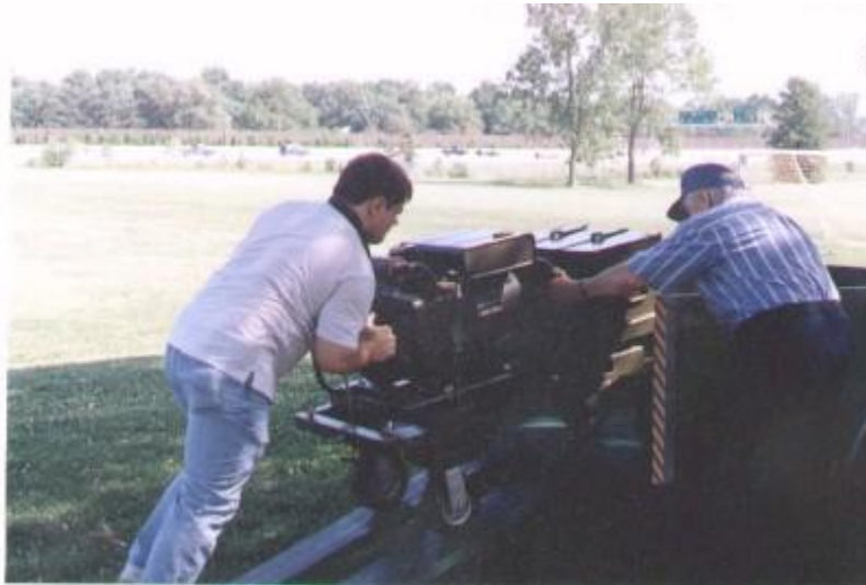
Photo 7: Where would we be without our reliable AC power? Mike N0MCG and Mac W0LQV unload the AC generator. Mac has been providing AC power for our FD operations since way before KCPL got in business!
